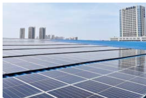
Solar power generation system installed at a factory
