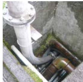
Before improvement Noise is caused by materials contacting the inside of the piping
