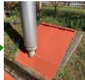
After improvement Sound absorption and insulation materials are installed A cover is also installed over the area where noise is generated
