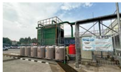
Cooling water tower and storage tank
